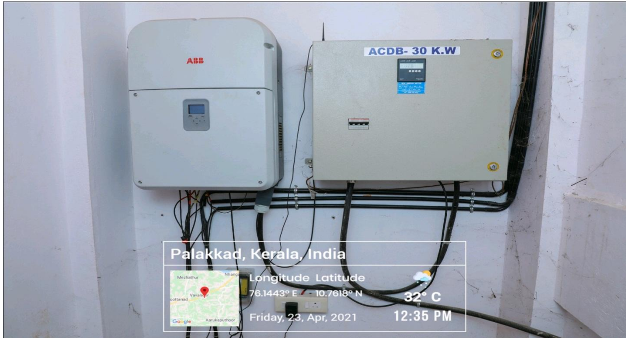
Grid tied inverter & Solar DB
