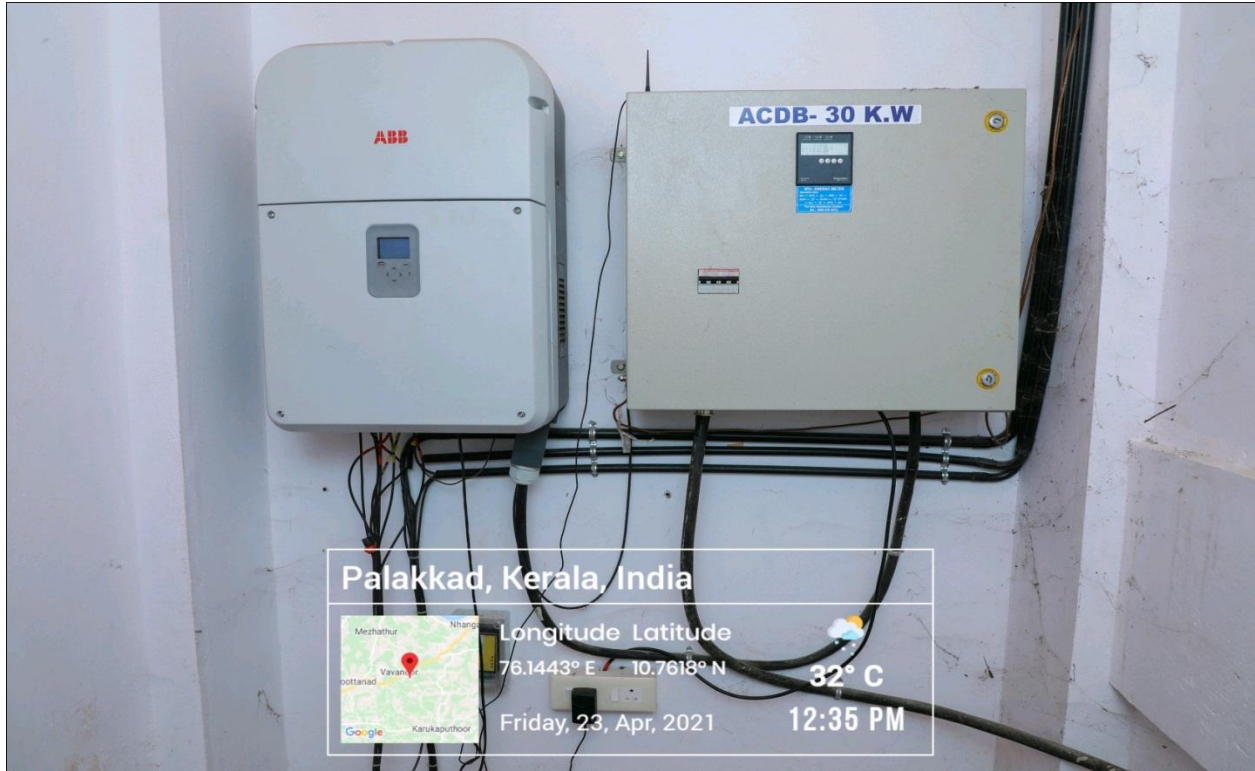
Grid tied solar inverter & solar DB
